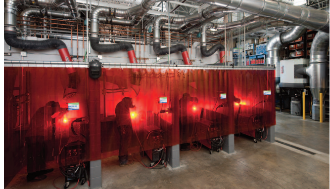
The weld fume control system removes and extracts welding fume at the point of welding and transports it via ducts to a central location for filtration.
