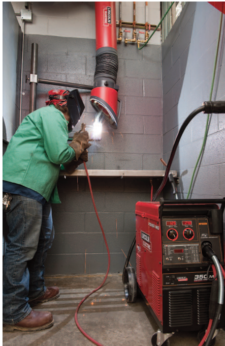
Fifteen welding booths are equipped with a variety of welders and weld fume control from Lincoln Electric.
