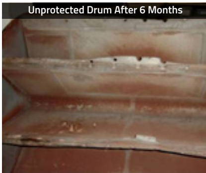
Vane pockets are damaged by wear and corrosion and must be replaced.
