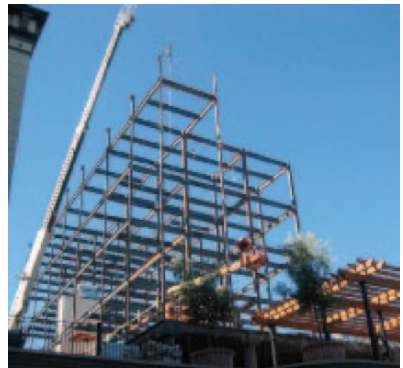
Erection is quick using ConXtech's Simmons Moment Resisting Space Frame (SMRSF) system.
