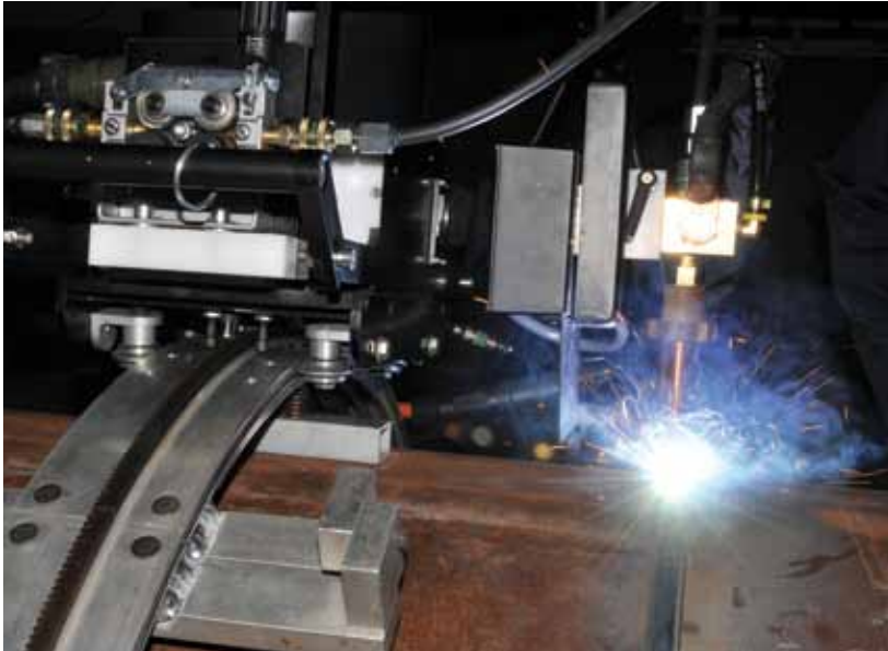
By using a Bugo Piper-Bug with solid wire STT for the root and gas-shielded FCAW for the fill passes, 30 joints per day can typically be achieved.
