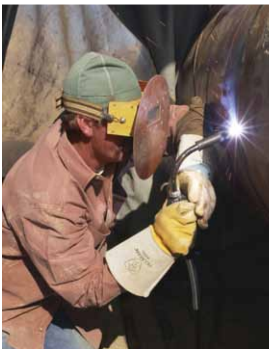
The use of Lincoln's STT GMAW solution not only offers productivity advantages, it also obviates the need to remove 'wagon tracks' associated with an SMAW root. This can significantly reduce the amount of rework required.
